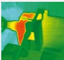
Motor: Bearing Problem
